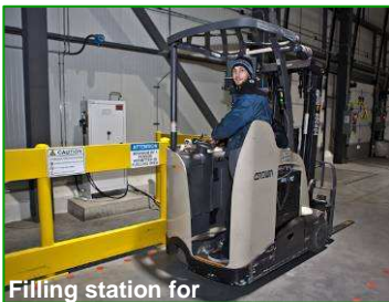
Filling station for Hydrogen powered forklifts Walmart - Canada
