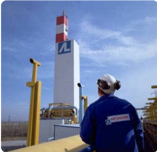
Air Separation Unit (ASU)
