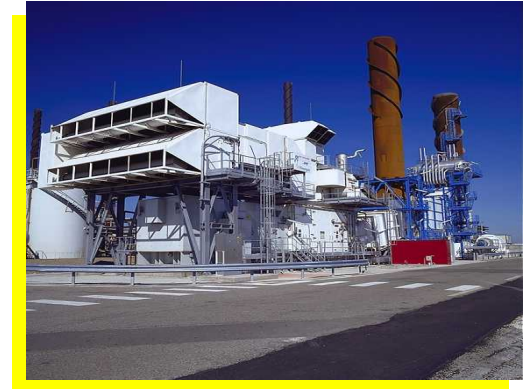
19 Industrial Cogeneration Trains
