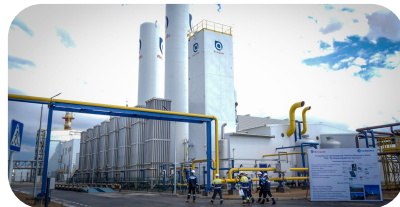
Nitrogen for SILLENO Petrochemical
